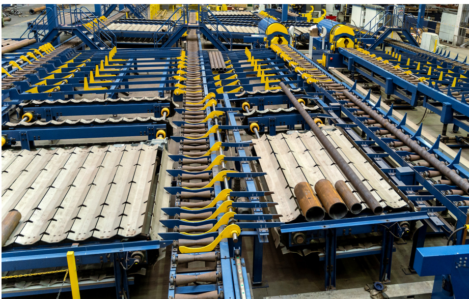
With an automated transport system no machine or worker has to wait for material, but can work continuously.
